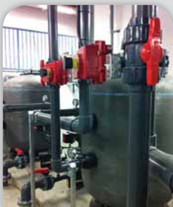
PVC ball and butterfly valves in penguin exhibit water treatment system
