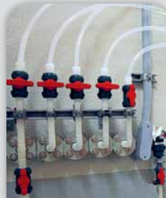
ChemFlare™ System (valves, fittings, tubing) for sodium hypochlorite in a water treatment plant
