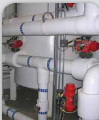
Pneumatically actuated PVC butterfly valves in walrus exhibit water treatment system
