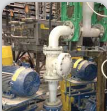
PVDF pipe, fittings and valves for sulphuric acid in a lithium processing plant
