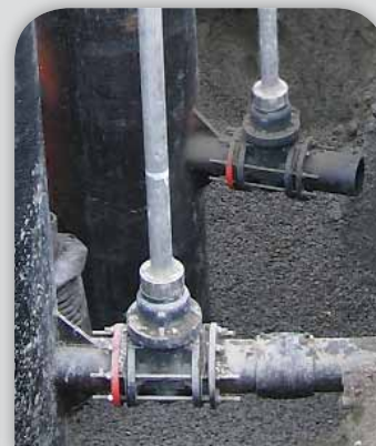
8" PVC gate valves with stem extensions for a landfill leachate collection system
