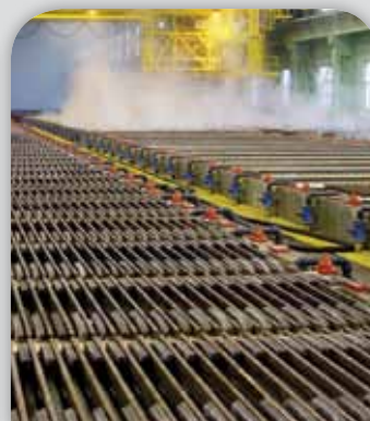
Butterfly and diaphragm valves for sulphuric acid in a copper and zinc electrowinning plant
