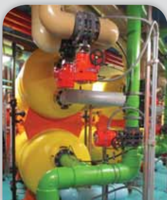
Electrically actuated PVC butterfly valves in aquarium sand filter system
