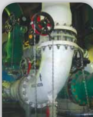
16" Polypropylene butterfly valves with chainwheel operators on a weak acid system in a sulphuric acid plant
