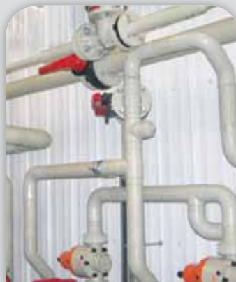
Butt weld Polypropylene pipe, valves and fittings for a ferric chloride system at a sewage treatment plant
