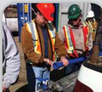
Blue PE piping for an underground compressed air system in a railway yard
